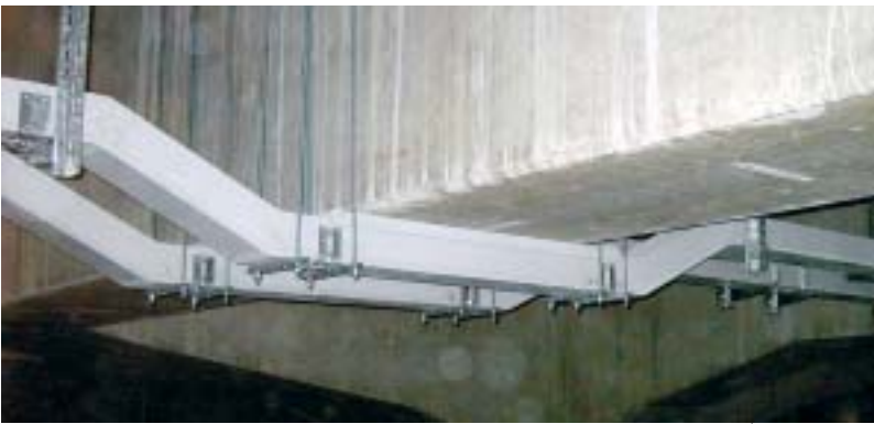
Suspended AESTUVER fire-resistant cable ducts
